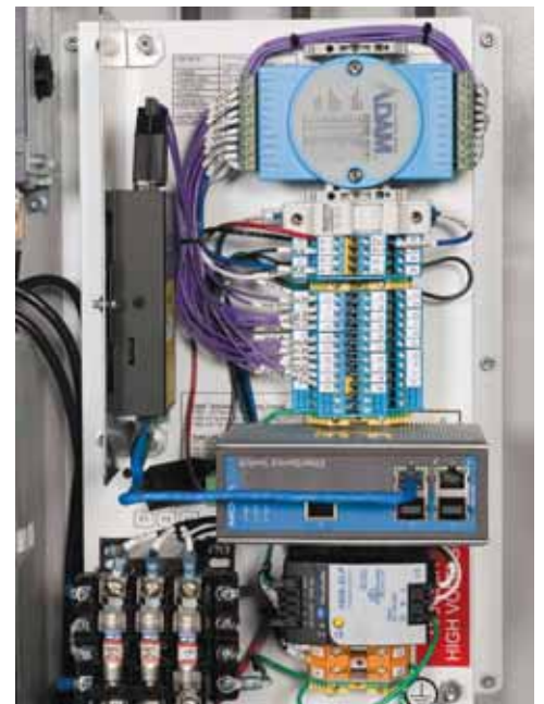
▲ A UL508A panel with integrated monitoring hardware.
